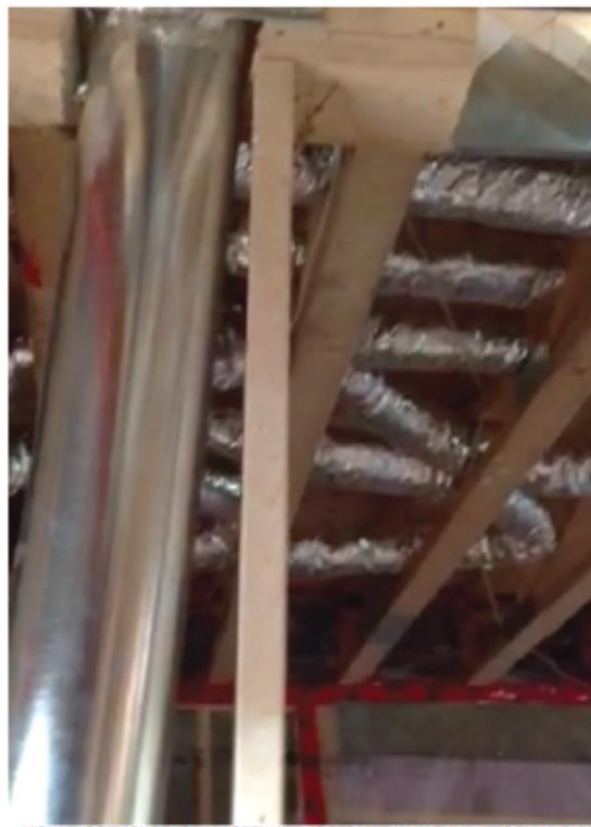
HIGH VELOCITY DUCTWORK IN OPEN WEB JOISTS VIRTUALLY ELIMINATES BULKHEADS*
